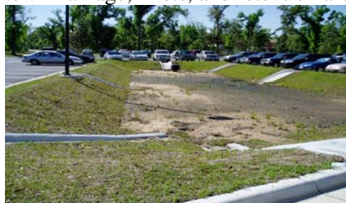
New Drainage, inlets, and retention area
